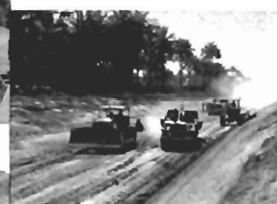
(top centre) Unloading caissons for Rio Nunez bridge foundation under construction in Guinea
