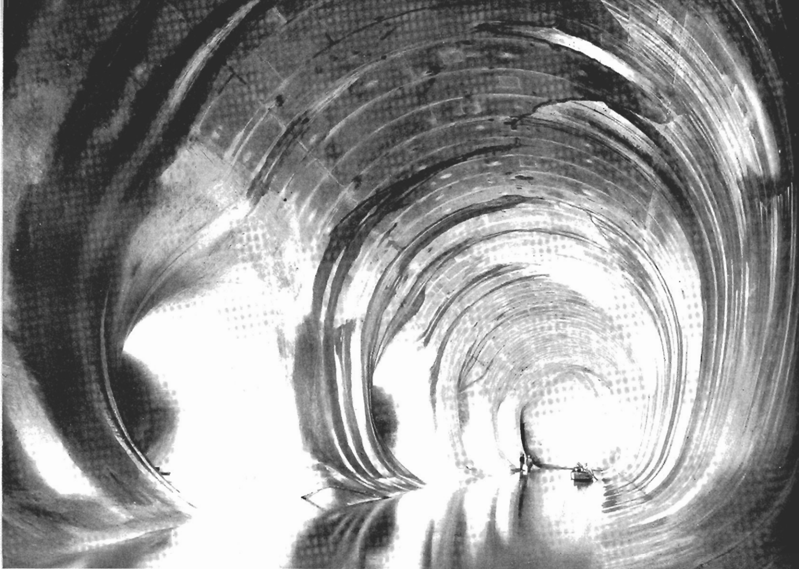
CHUTE-DES-PASSES. Inside the six mile main water supply tunnel showing the entrances to the penstocks on the left leading to the five turbines. This photo was taken prior to the opening of the control gates, and watering of the tunnel
