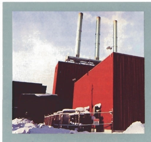
New electrostatic precipitator unit removes contaminants from Steelworks' sinter plant stack gases.
