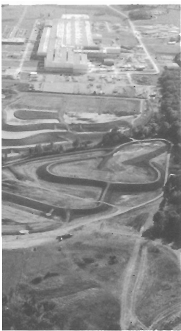
A new wetlands system for wastewater treatment, pictured here during construction last fall, is an economic and environmental success for Logan Aluminum Inc. in Kentucky. The 40-acre system naturally purifies water from the mill while aiding the local ecosystem.
