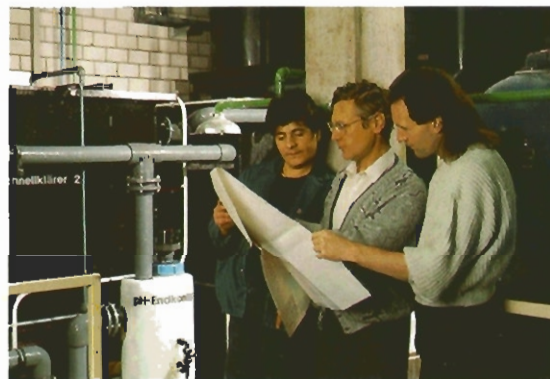
Bottom right: In Switzerland, engineers Angelo Terranova, Engelbert Müller, and Roland Müller check the installation of Rorschach's effluent control on a new annealing/pre-treatment line for foil packaging material.
