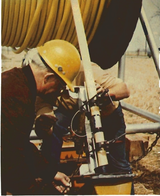
Above: Using Alcan designed techniques, high-energy joining of aluminum provides fast and economic installation of continuous coils of gas distribution pipe in the field.
