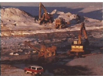
Heavy equipment moves into place at the banks of the Peace River in preparation for the laying of the pipeline.
