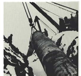
This large diameter 36 inch pipeline is lowered into place on Flathead Ridge in 1961 at the highest point (7,000 feet) on the Alberta California Pipeline.
