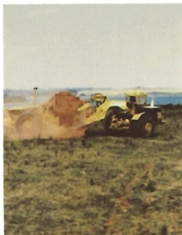
Earth movers take the first bites of Irish soil for construction at the Ringaskiddy site.
