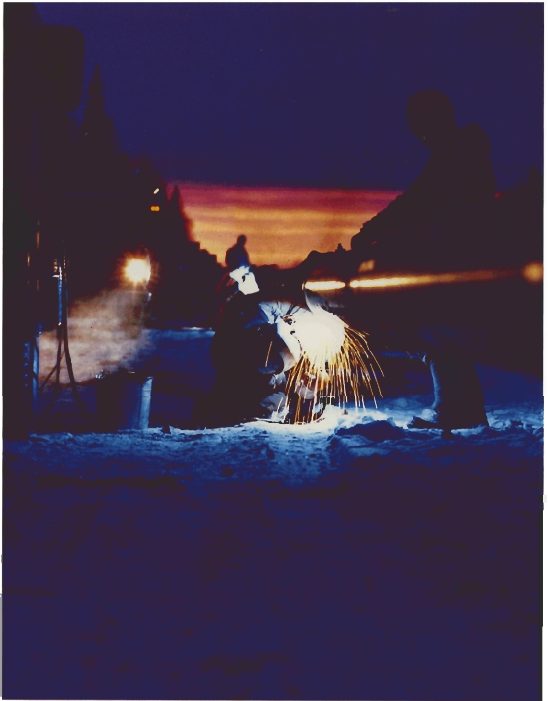
The setting sun is overpowered by the flash of a welder's arc on the Shell Canada Resources pipeline at Peace River, Alberta.
