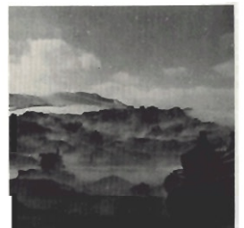
The morning mist provides an eerie quality to this platoon of bulldozers grading a creek embankment in 1962 on the Alberta-California pipeline right of way in the Porcupine Hills of southwestern Alberta.
