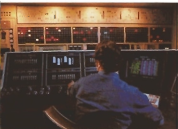
The nerve centre of the company's Cochrane plant is this ultra-modern control room which monitors controls all vital plant functions.
