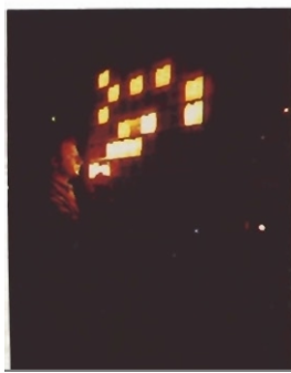
This central alarm panel at the Crossley Compressor Station No. 1 monitors a wide variety of functions.
