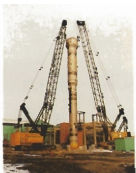
In 1982, construction began on the second plant expansion. One of the two demethanizer towers is being raised.
