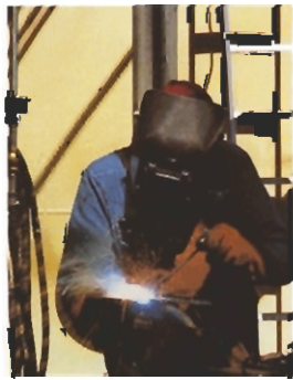
This welder was one of many workers who laboured on the Cochrane plant's second expansion, which took place in 1985.
