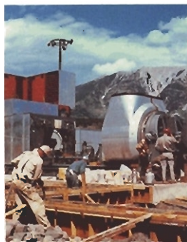
Construction began in 1967 to increase the compressor capability of Alberta Natural's Crowsnest Compressor Station No. 1
