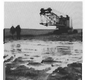
The first crane moves into place to begin construction of the new Cochrane gas plant in 1969.
