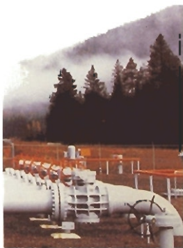
These valve assemblies are a portion of the Kingsgate Meter Station on the International Border.
