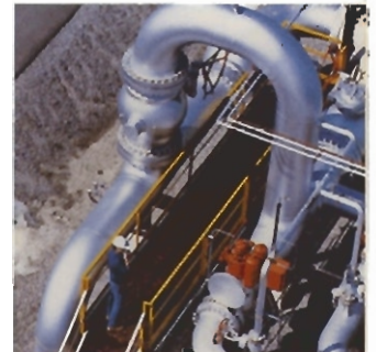
An employee at Alberta Natural's Cochrane liquids extraction plant is dwarfed by large diameter pipes carrying natural gas.
