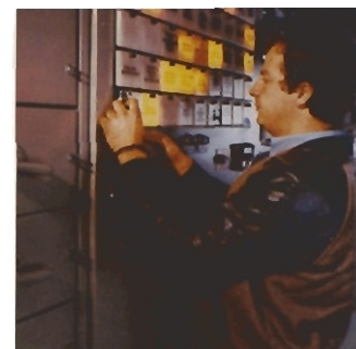
Senior Electrical Technician Michael J. Ondrus monitors the compressor alarm panel at Alberta Natural's Compressor Station 1 in the Crowsnest Pass.
