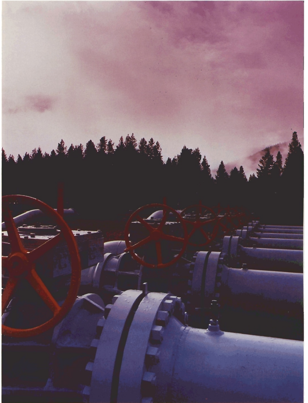
Portion of the Meter Station complex located near Kingsgate, British Columbia – the final Canadian point in the export of natural gas to United States markets
