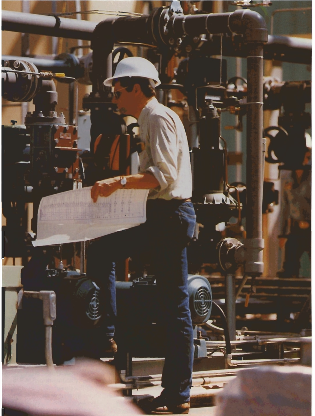
Final inspection of the 40 Cwt sulphur removal facility prior to its commissioning following the Cochrane liquids extraction plant expansion
