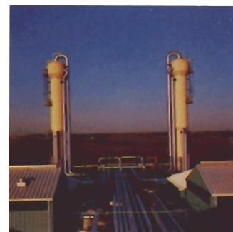
Two demethanizers dwarf a portion of Alberta Natural's Cochrane liquids extraction plant which houses the two turbo-expander trains, an integral part of the plant's recent major expansion.
