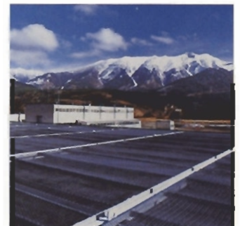
Alberta Natural's Grousenest Pass compressor station develops 40,000 horsepower from three compressors.
