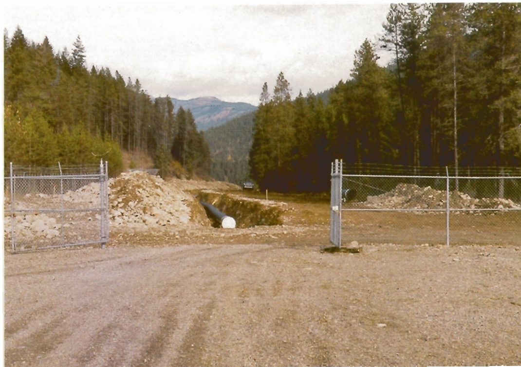
View of pipe prior to connection at the Kingsgate meter station.
