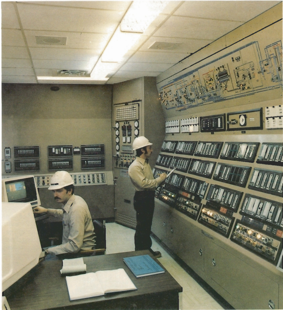
View of Cochrane Plant control room showing operator at computer control consoles monitoring operating conditions.
