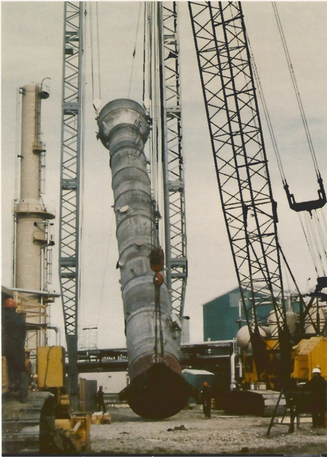
De-methanizer process tower being raised into position at the plant site. This stainless steel column is 111 feet in length, 8 feet in diameter and weighs 70 tons.
