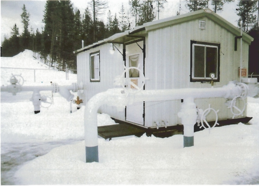
View of the new East Kootenay Meter Station near Yahk, British Columbia.
