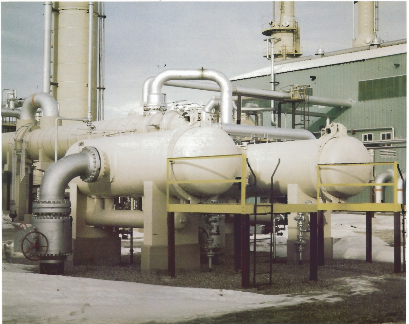
View of new inlet gas filter installation at the Cochrane liquids extraction plant.
