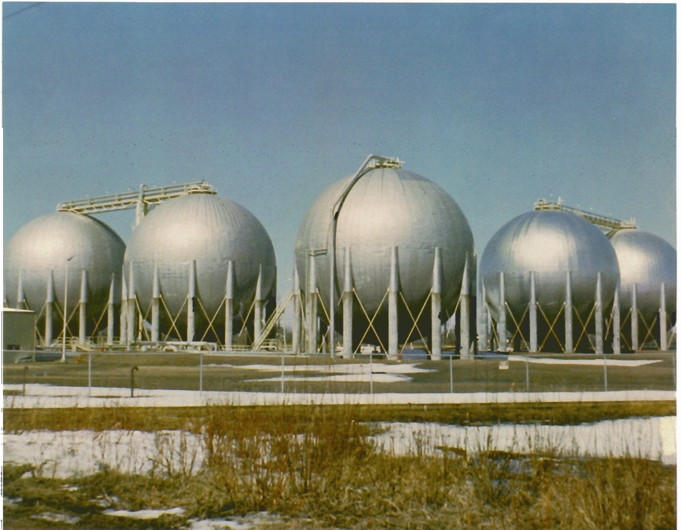
View of the storage facility at Superior, Wisconsin which holds the Cochrane plant liquid products at time of transmission transfer between pipeline systems.
