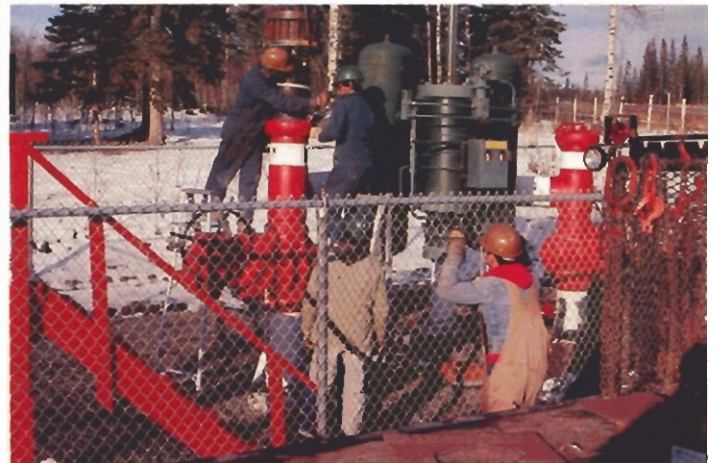
Transient wave monitoring, line break detection study
