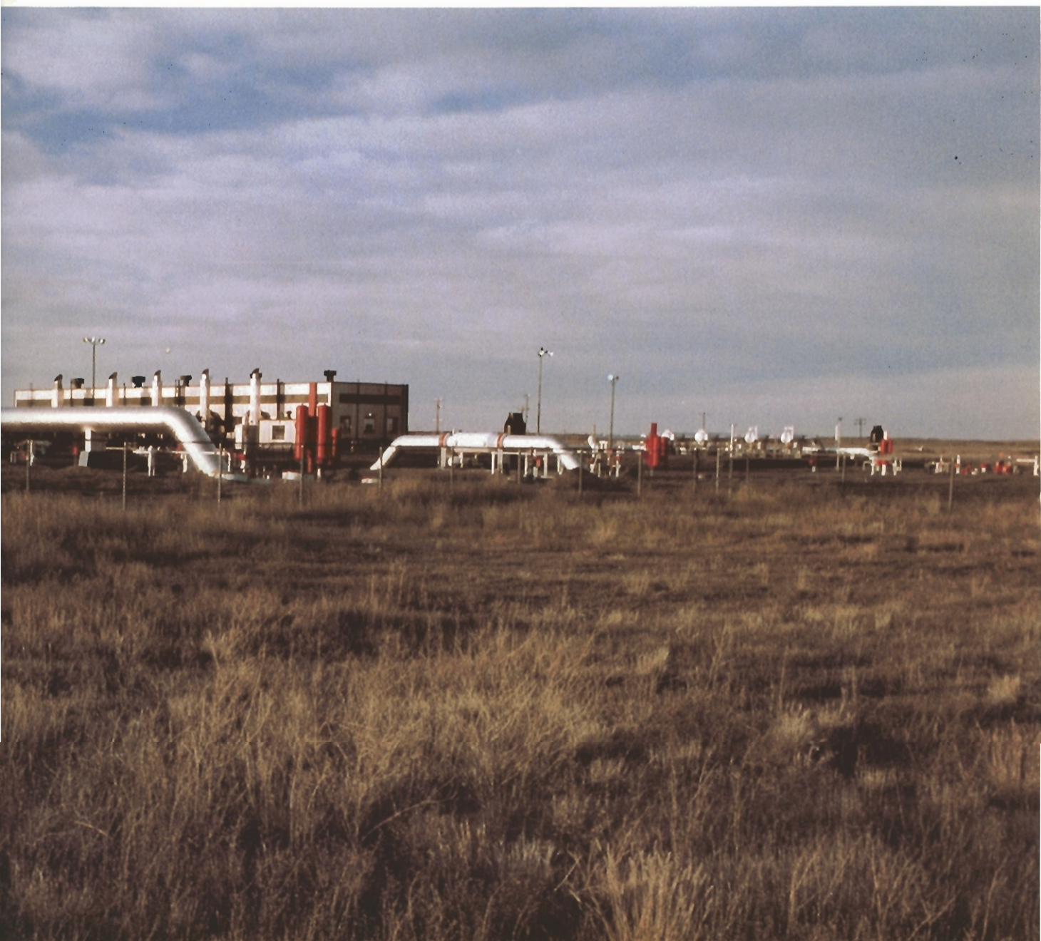
The Company's largest compressor station, Princess Alberta.
