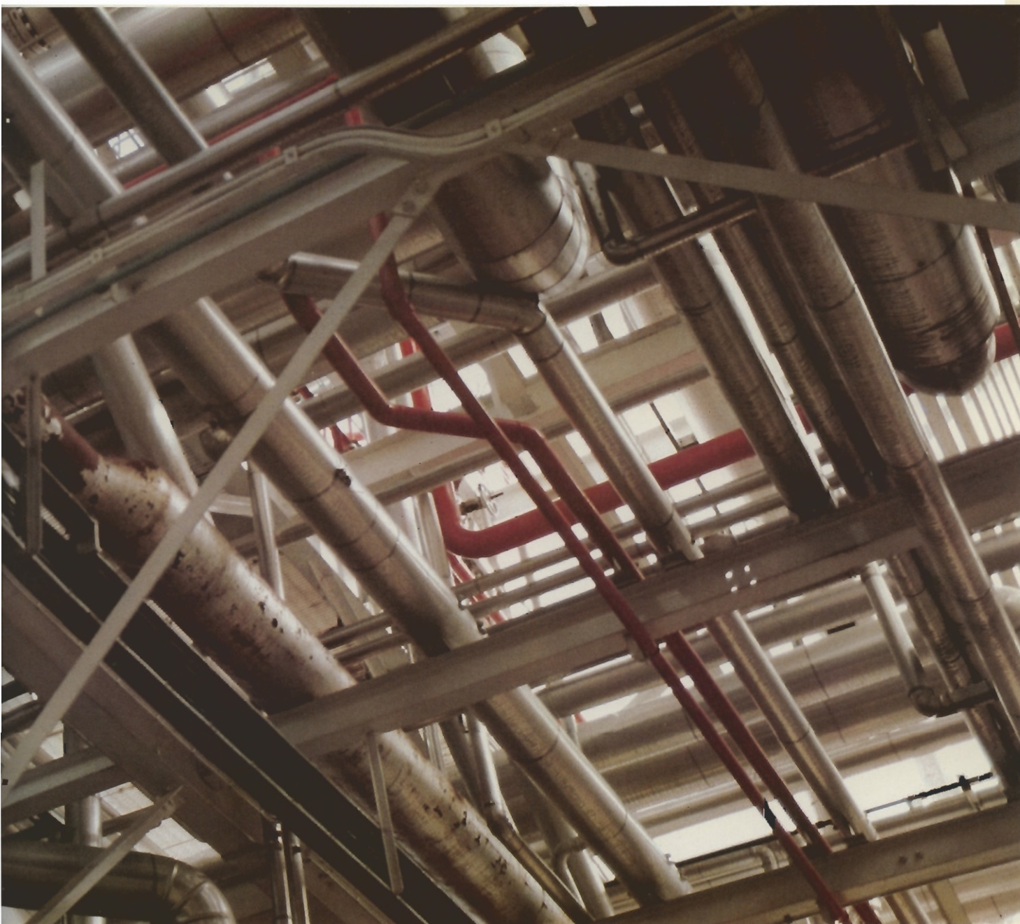
Intricate networks of pipe form an integral part of the methanol plant
