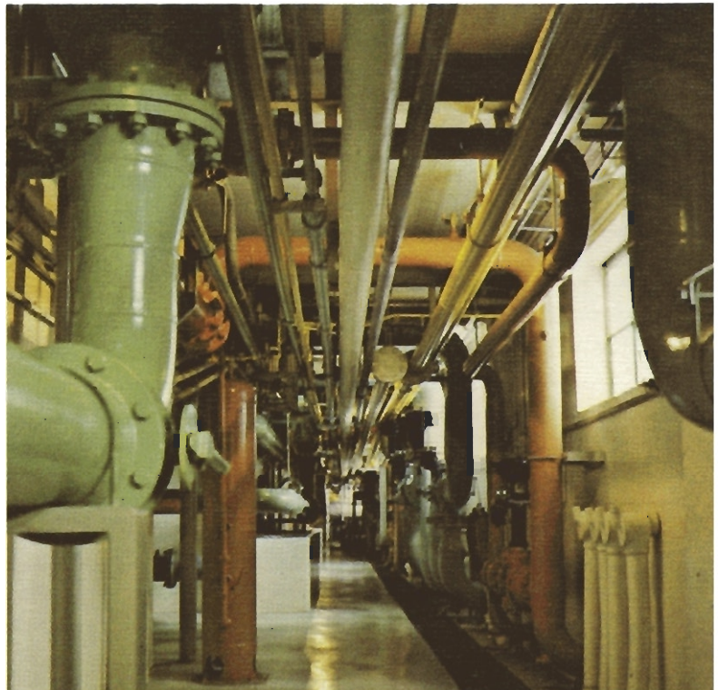
Hundreds of feet of "plumbing" form an important part of the Company's large compressor station at Princess.
