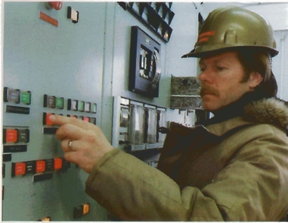
Interior of pipeline control unit
