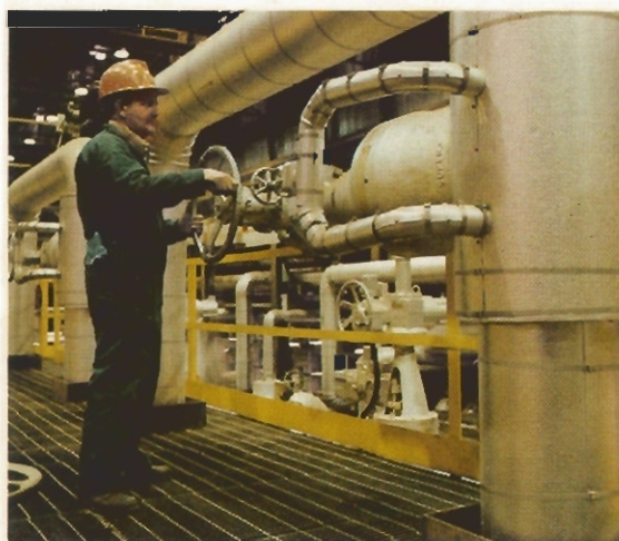
Above: Interior of Utilities Plant
