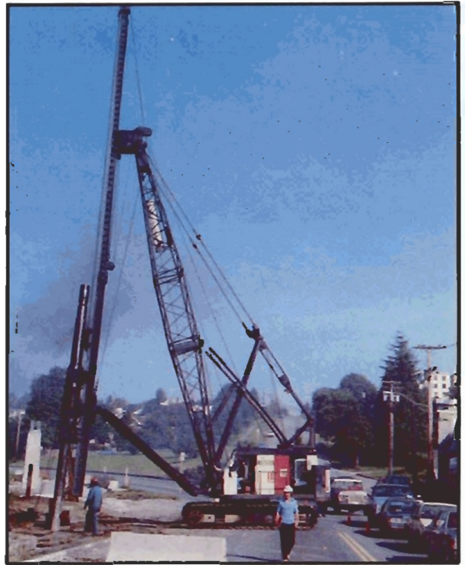
Western Caissons drives steel piles over 150 feet deep to support the ALRT transportation system which will run from New Westminster to downtown Vancouver.
