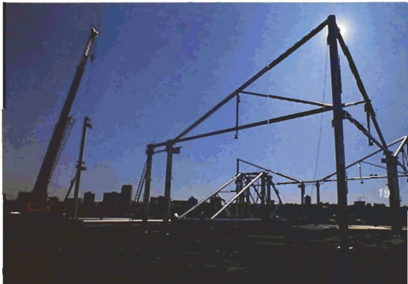
Coast Steel Fabricators manufactured and is erecting the prototype building which will be used as the Exhibitors' Pavilion for Expo '86 in Vancouver.
