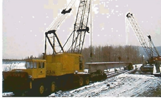
Jensen & Reynolds erecting 135' long, 82-ton concrete girders at Hess Creek, Alaska, for their bridge project 30 miles south of the Arctic Circle. The transportation and erection of the girders represented the longest and heaviest loads ever moved over the North Slope haul road.
