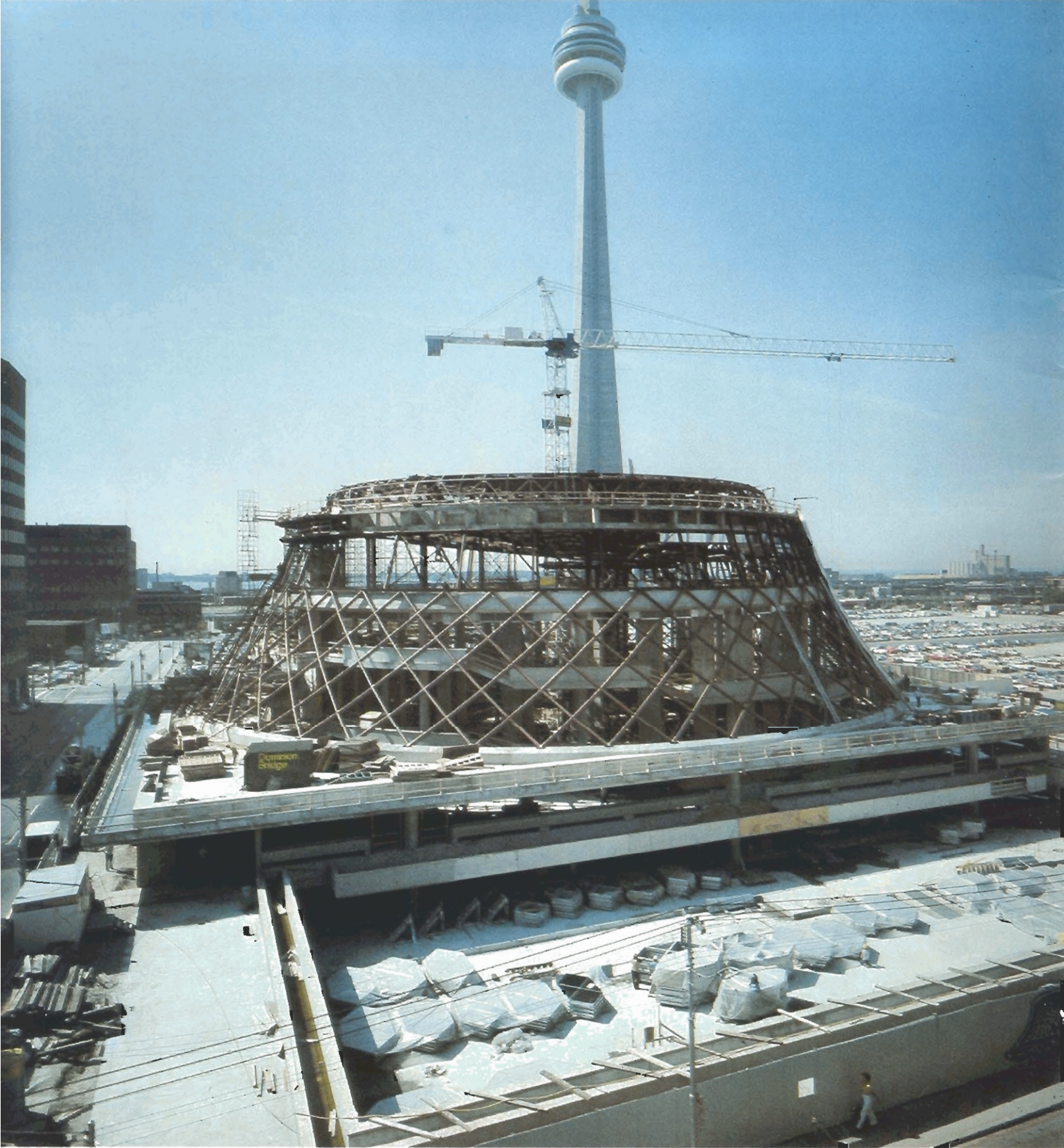
Beer Precast are erecting ceiling panels, roof panels and balustrades for the magnificent new Massey Hall in Toronto.
