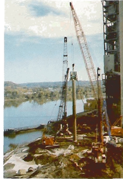
Western Caissons install 5 foot caissons 90 feet deep for the Philip Sporn power plant in West Virginia.
