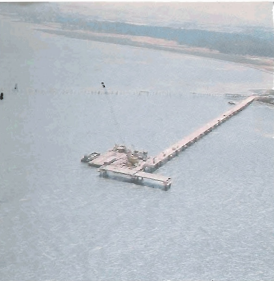
Jensen & Reynolds constructed the fishing wharf at Point Pinole in the San Pablo Bay area north of San Francisco.
