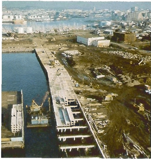
The coast guard dock near Dallas Road in Victoria, B.C. was constructed by Greenlees Piledriving in 1977
