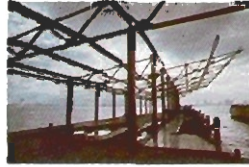
▲ Coast Steel Fabricators fabricated the steel framing for the Burrard Inlet Ferry Terminal building in British Columbia.
