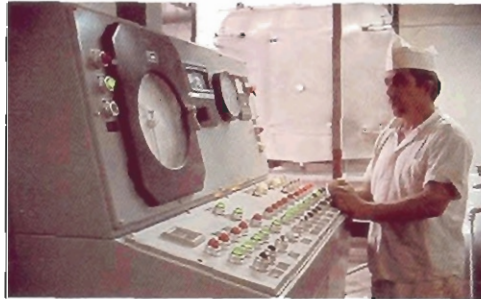
Automatic control panel in Research Food's plant in Toronto.
