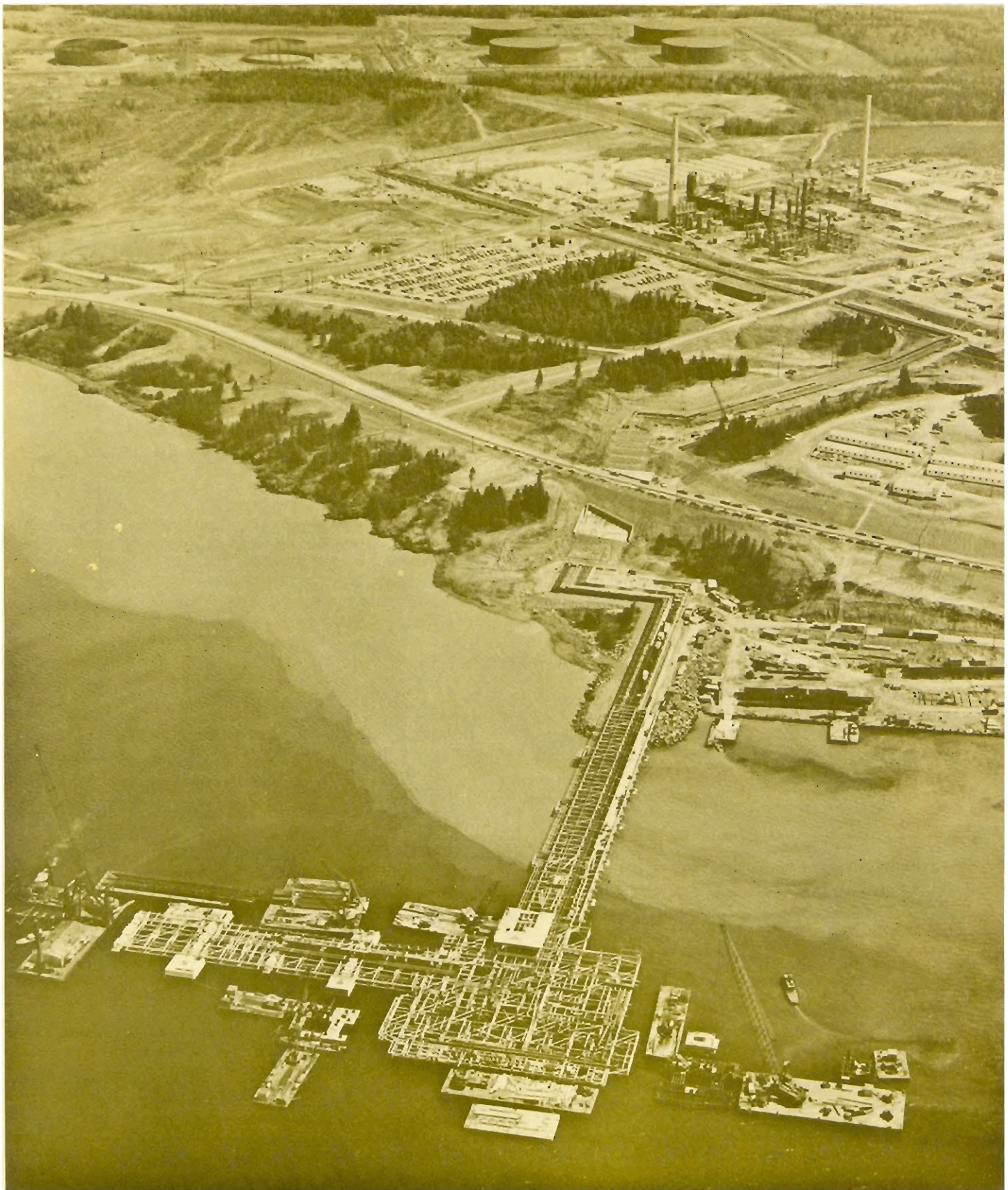
Thrusting 750 feet from shore, in the Strait of Canso, is the 17 million dollar dock being built to serve Gulf Oil, Canada's new 60 million dollar refinery, nearing completion of Point Tupper, Nova Scotia. The dock, which provides a water depth of 100 feet, will be the first in the Western Hemisphere, capable of handling the world's largest ships. Deep piles to support this dock were socketed into bedrock up to 200 feet below water surface, by Western Caissons for Pits Construction Limited, general contractors for the project.
