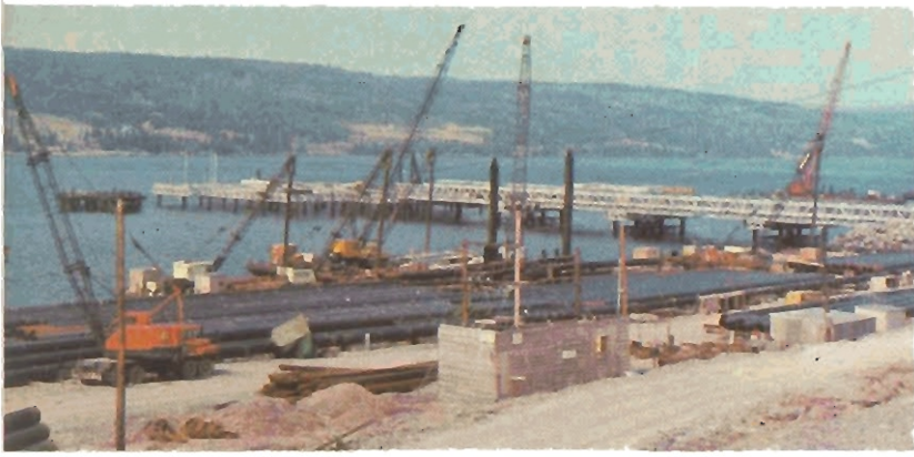
Western Caissons drilled piles to almost 200 feet below ocean level, for Gulf Oil's new Super Tankers Port in Conso Strait, near Point Tupper, Nova Scotia
