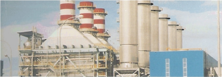
Grati Power Plant – Indonesia
