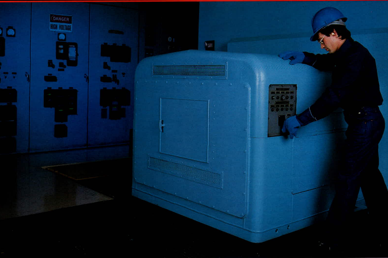
Gord Hannah (above) checks turbo generator #1 as it goes into service following a maintenance overhaul.
