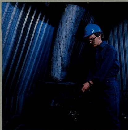
Martin Cutler inspects rebuilt boiler #2 in the utilities plant prior to start-up.
