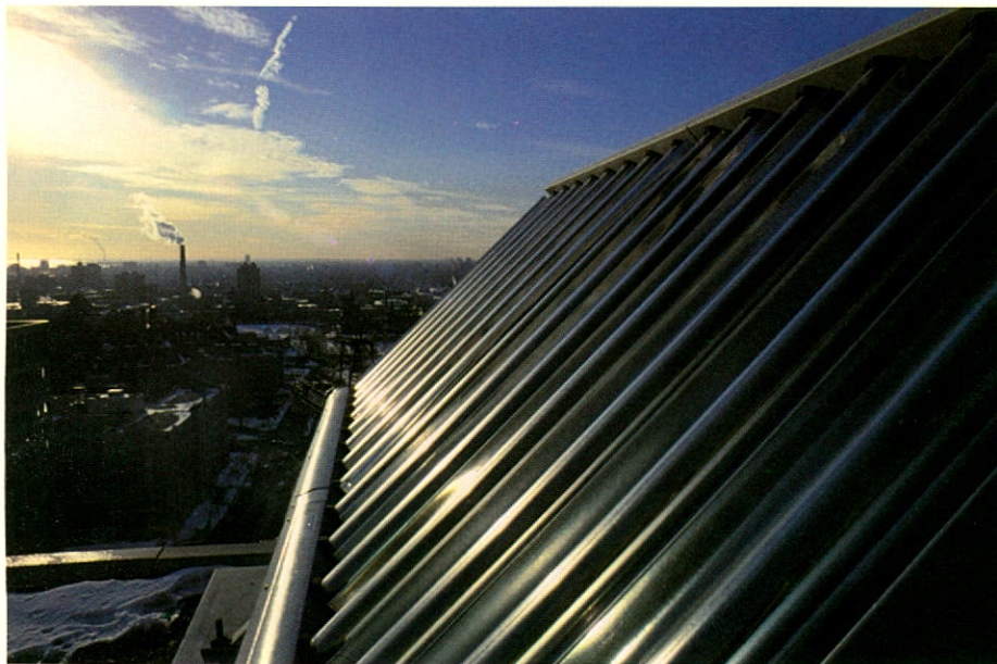
Solar panels on the roof of the Sunoco Group's downtown Toronto office building were installed by Solartech, a company in which Suncor has a 15 per cent interest. The panels provide heat for hot water.
