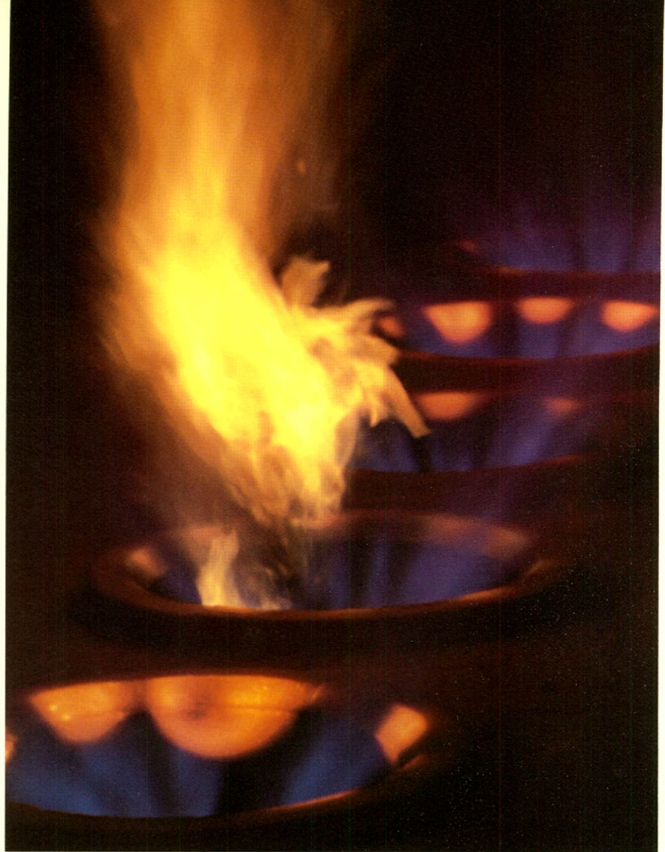
Burners in one of the pretreaters at Suncor's Sarnia refinery. Pretreaters remove impurities in manufacture of high-quality gasoline. Refinery operated at 86 per cent of rated capacity in 1980.
