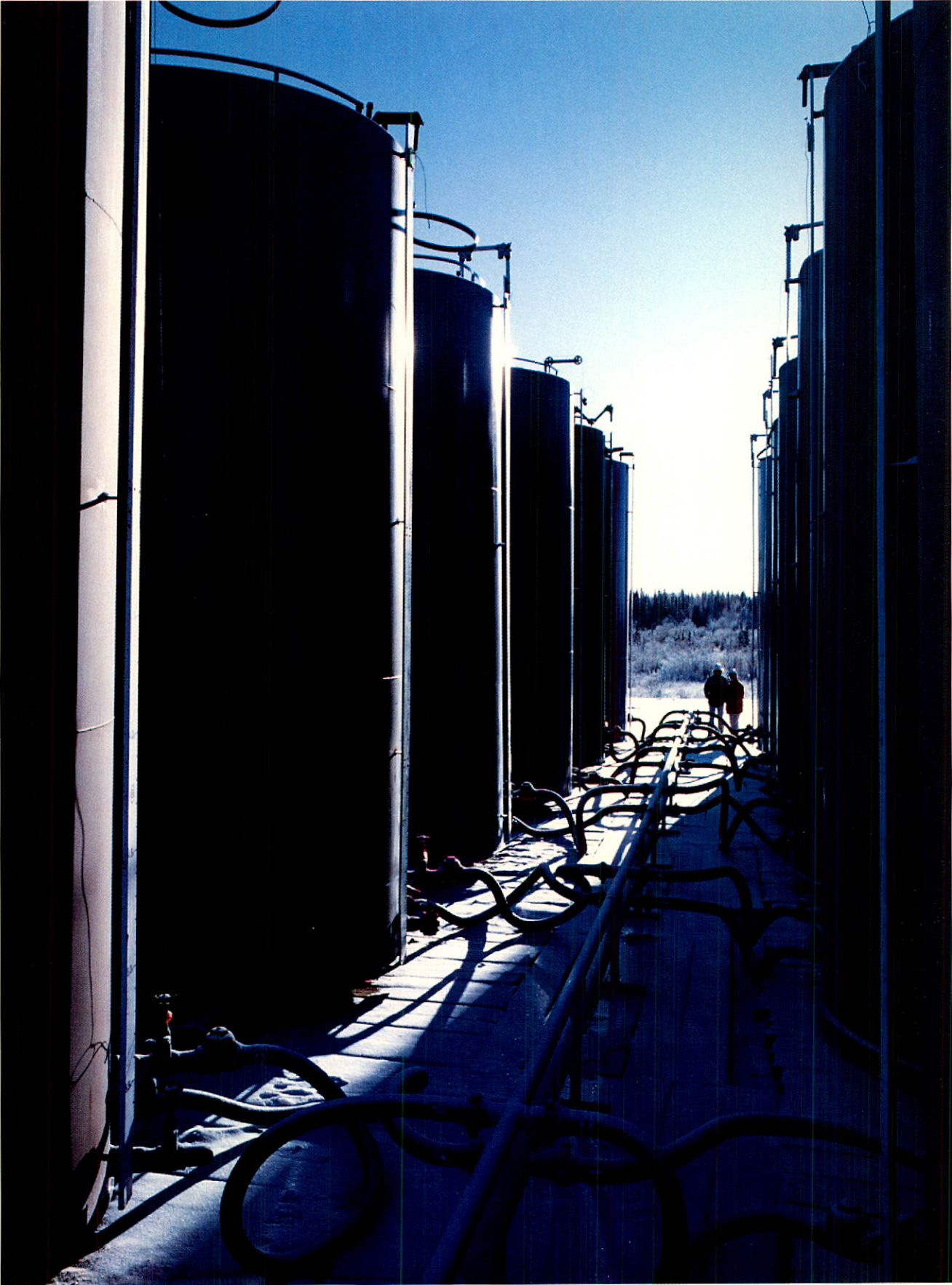
Temporary crude oil tank farm used in production testing, located at 10-31-108-6 W6 in the Rainbow Lake area.
