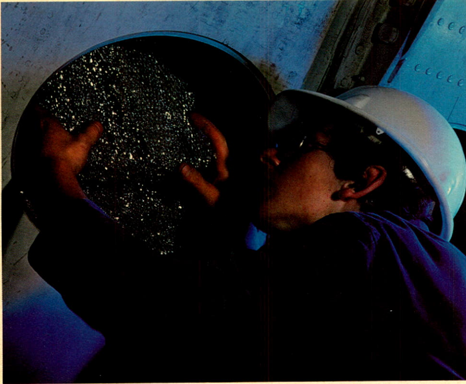
Installation of specially shaped batts of Explosafe foil around complex internal fittings in wing of A-10 aircraft.
