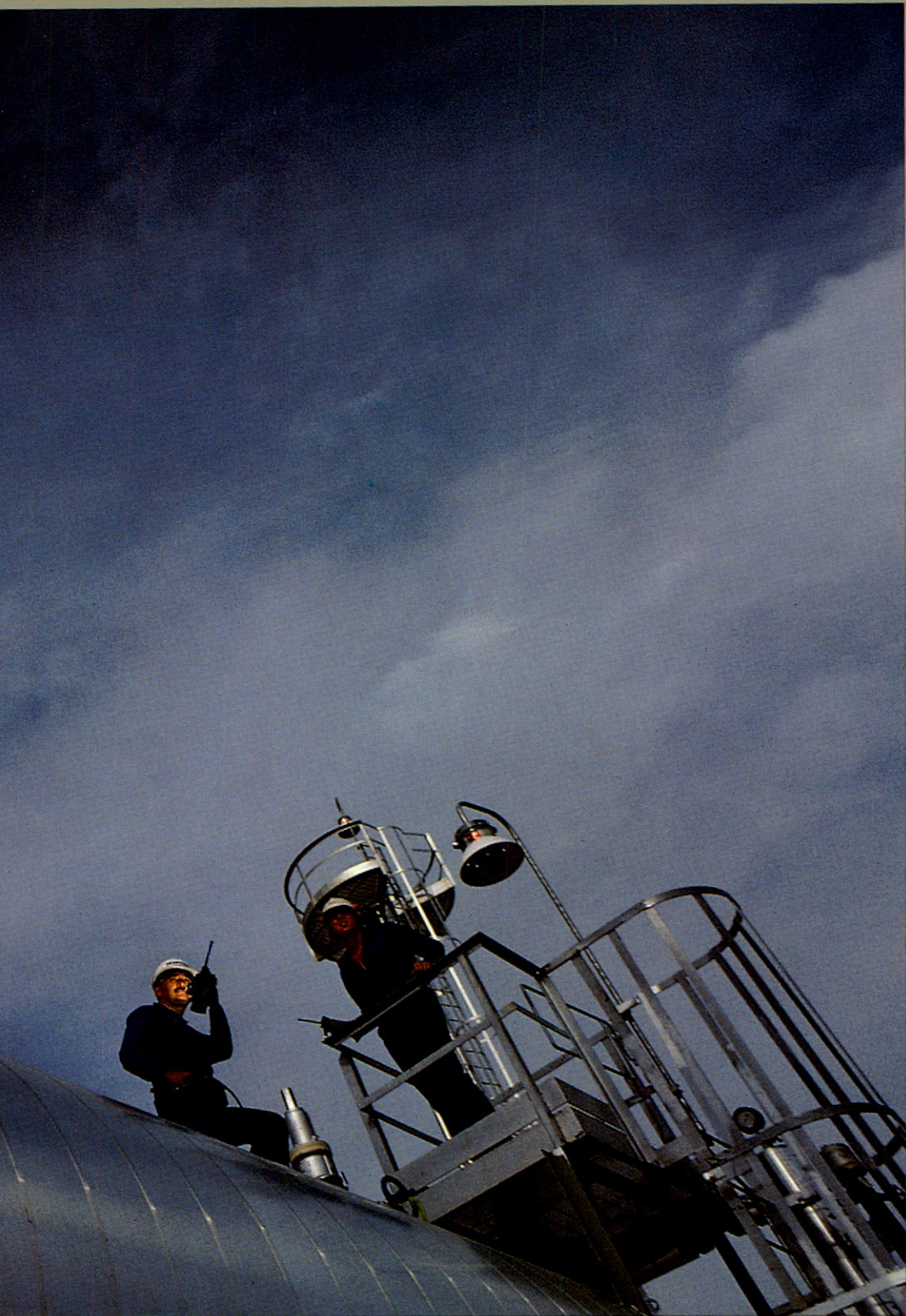
Norcen personnel supervise start up of the Company's new gas liquids extraction plant in Fort Saskatchewan.
