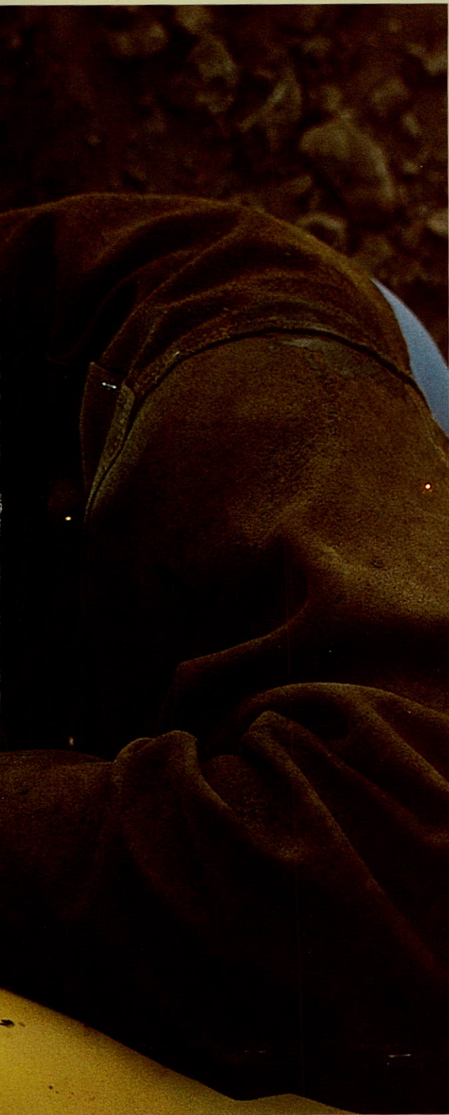
Laying new pipe in Picton, Ontario. One of the many projects, assisted by the Distribution System Expansion Program, undertaken in 1983 by Northern and Central Gas to connect additional customers.
