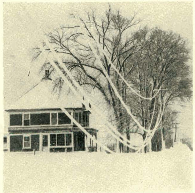
These sleet-laden wires, though badly sagged, are still in service.
