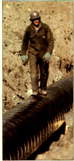
Phase 1 right-of-way wends its way south (left) near Nanton, Alberta. Workman (above) makes a visual check of the newly-installed line.
