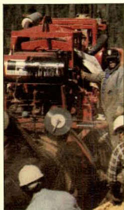
Coat and wrap machine (above) operates on the western leg in British Columbia, and welding crews (right) prepare to add another 24.4 m (80-ft.) section of pipe to the Alberta portion.
