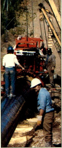
Executives (far right) of companies involved in the project spoke at commemorative weld ceremony. Coat and wrap operation (above) progresses on 914 mm (36-in.) pipe.
