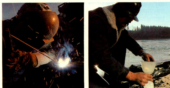
The past year was unusually active, with construction proceeding on small laterals as well as large-diameter loops and mainline. Environmental monitoring is carried out on a continuing basis.
