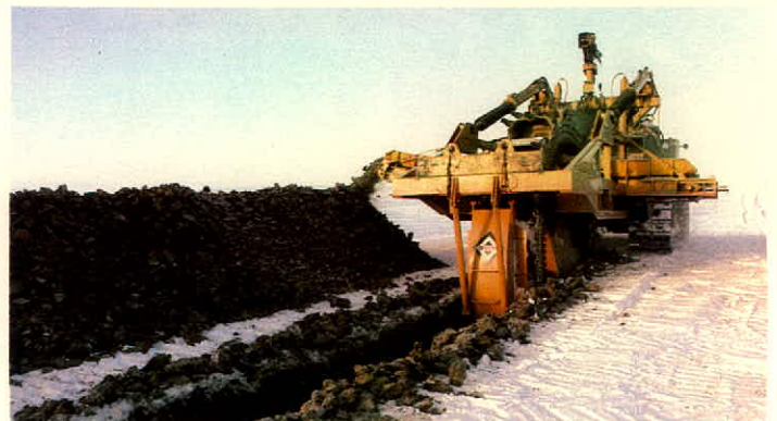
Phase I construction through southeastern Alberta and arctic testing of a new ditching machine were among 1981's highlights in the Natural Gas Transmission sector.
