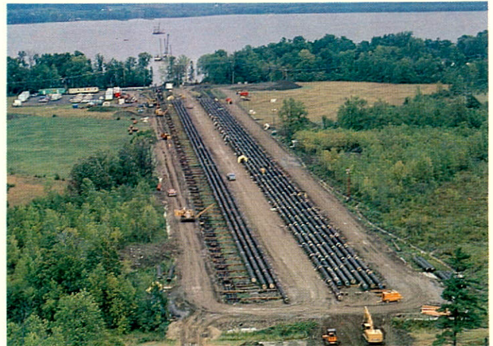
Trans Québec & Maritimes' Ottawa River crossing was a first step toward the connection of markets east of Montreal to domestic supply.
