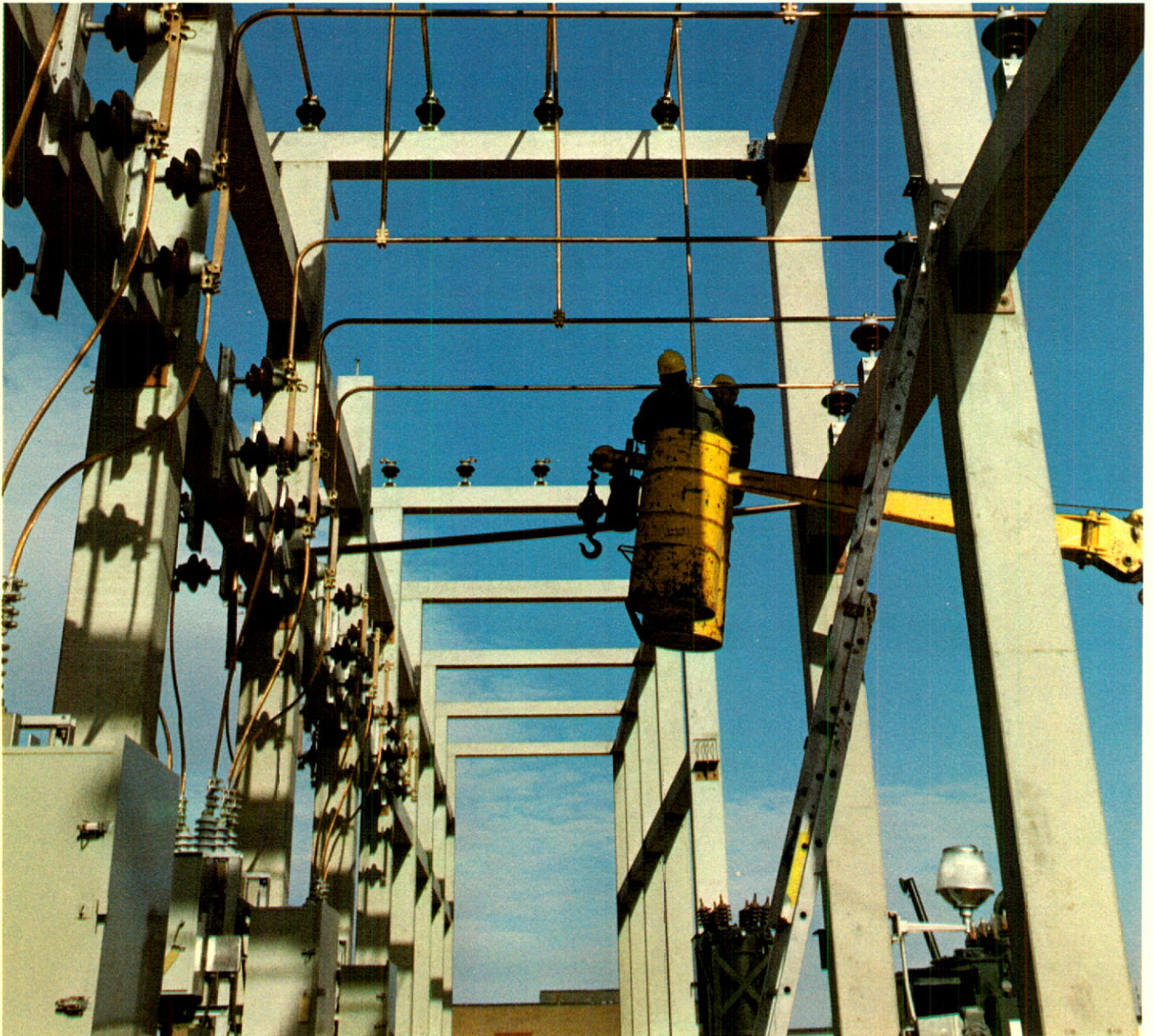
New type of distribution substation at Granby
