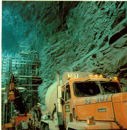
Concreting the plug in one of the two by-pass tunnels at LG-2.
