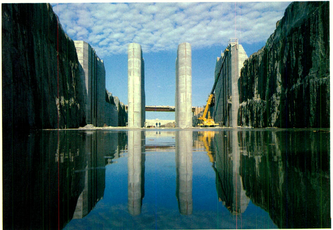
Spillway canal and pillars for spillway gates, EOL diversion project, James Bay region. The Eastmain River is diverted through this canal during construction of dam OA-11.
