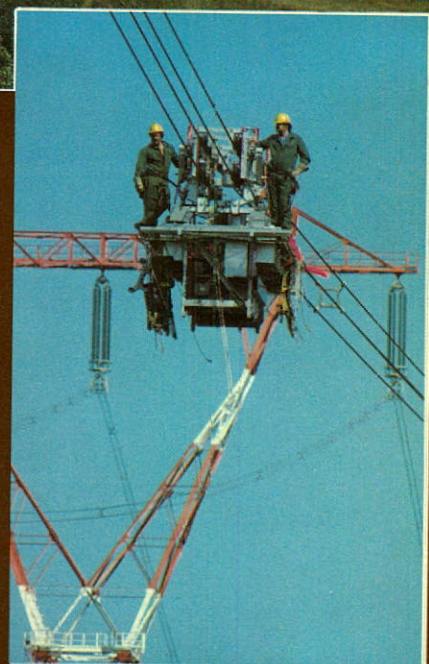
Transmission lines crossing the St. Lawrence River.
