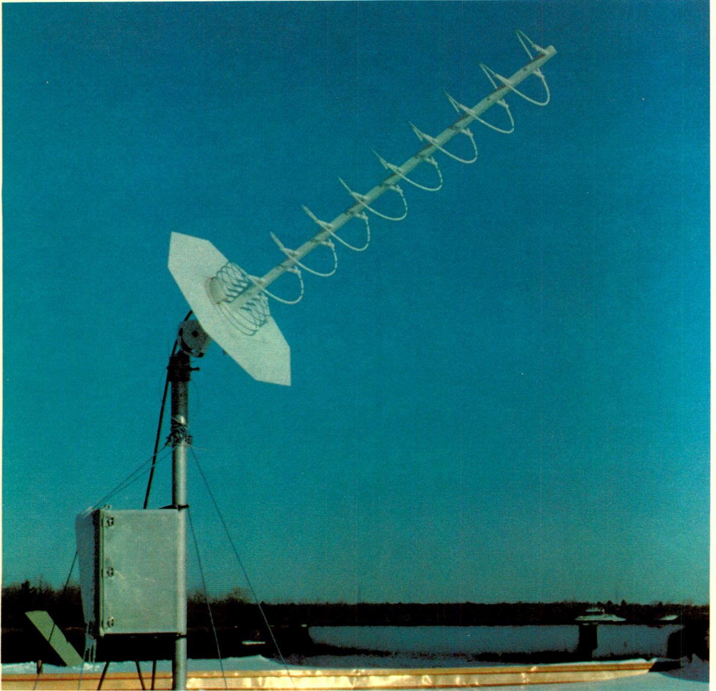
Microwave antenna at the IREQ laboratories.
