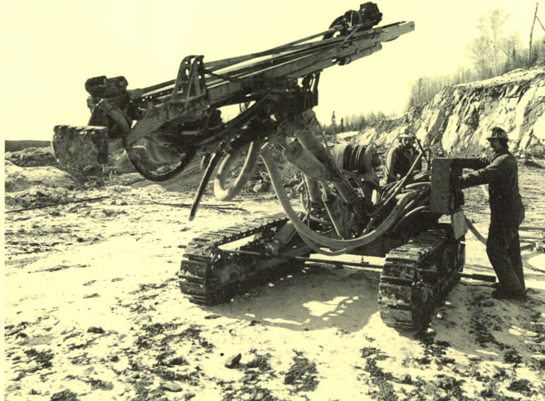
Miners moving Air Track Drill to new set up location at La Mine Doyon open pit, Quebec.
