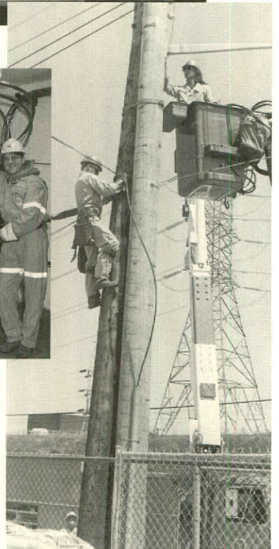
Improving the continuity of the power supply.
