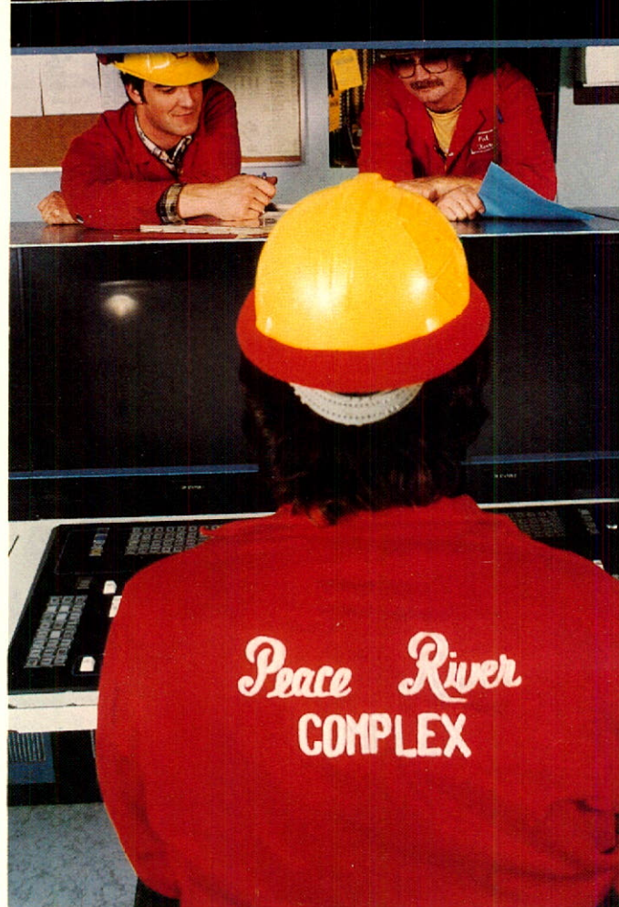
Duncan Cook and Pat Kerr with operator Bill Walsh in the technologically advanced control room which adjusts pressures and temperatures at the Peace River in-situ oil sands project.
