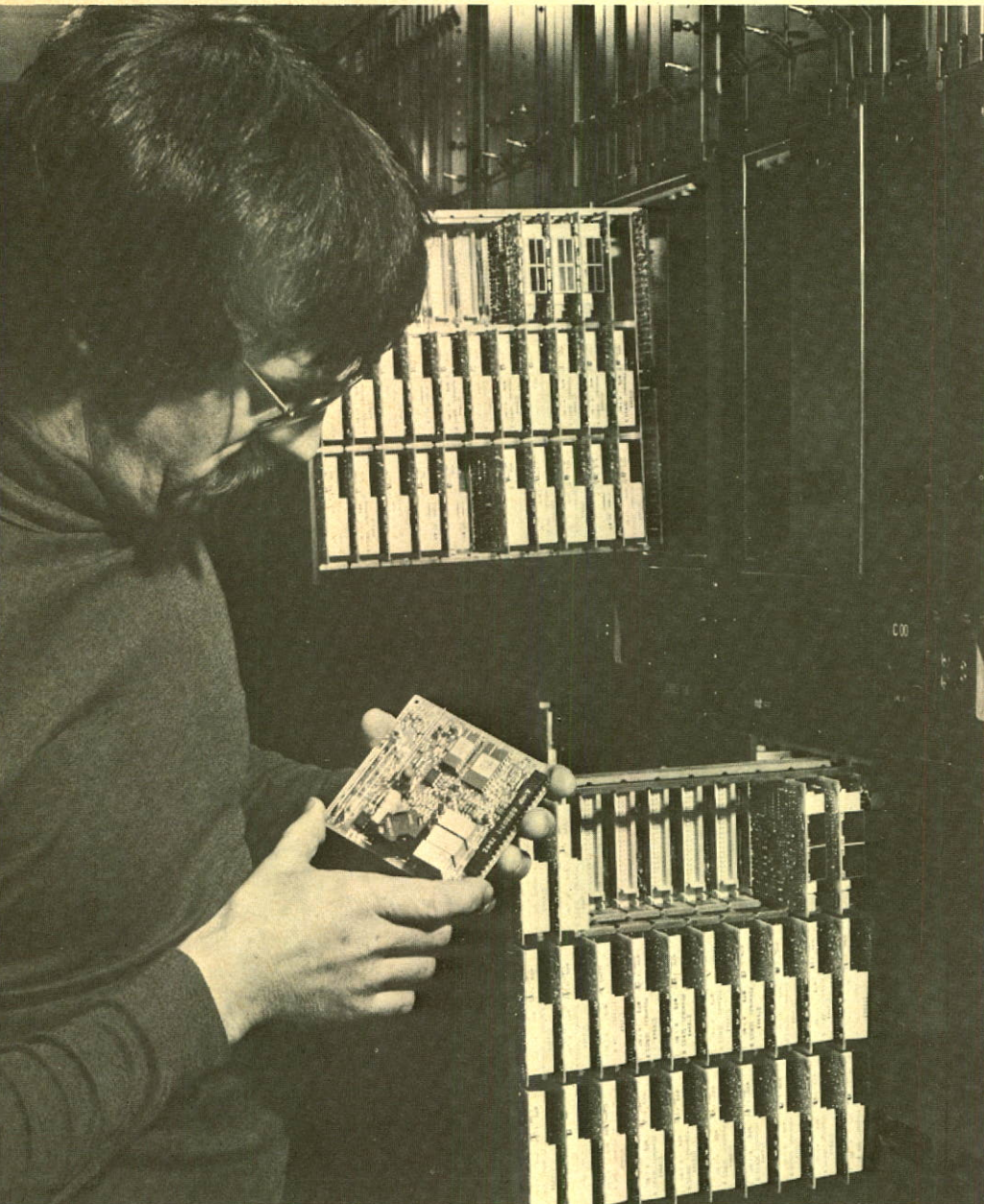
Digital switching equipment being installed in the Bridgewater office.
