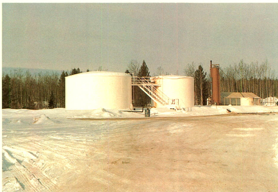
3,000 barrel storage tanks at the main Edson terminal connected to the Peace River Pipe Line.
