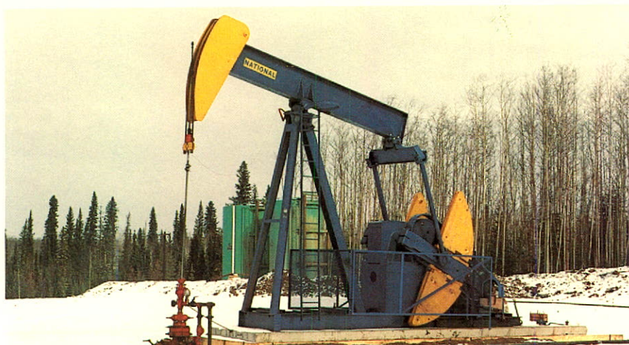
Pumping facilities at Otter 3-4.
