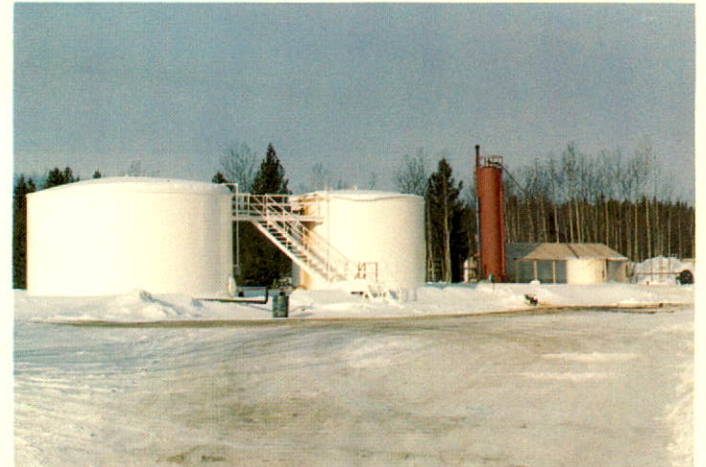
3000 barrel storage tanks at the main terminal connected to the Peace River Pipe Line.
