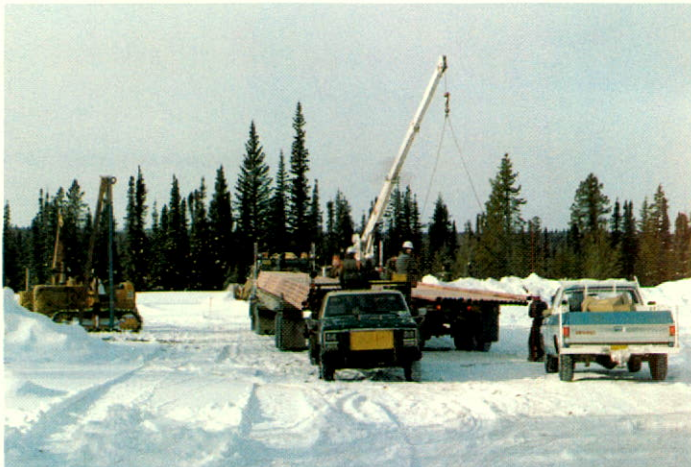
Offloading coated line pipe for a flowline from the satellite battery to the main terminal.
