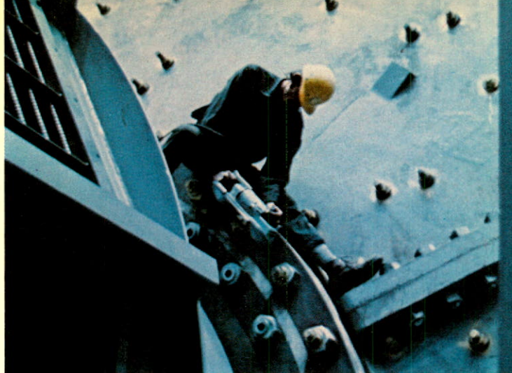
Lornex: A bolt is tightened on a giant autogenous mill just prior to start of production.
