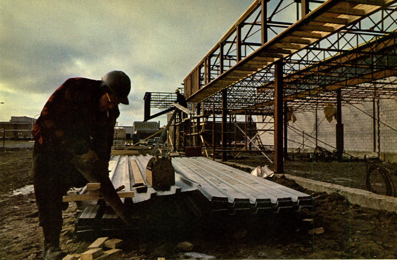
Silhouetted against overcast sky, construction worker prepares material for use in Atlas Alloys' new Montreal service centre.
