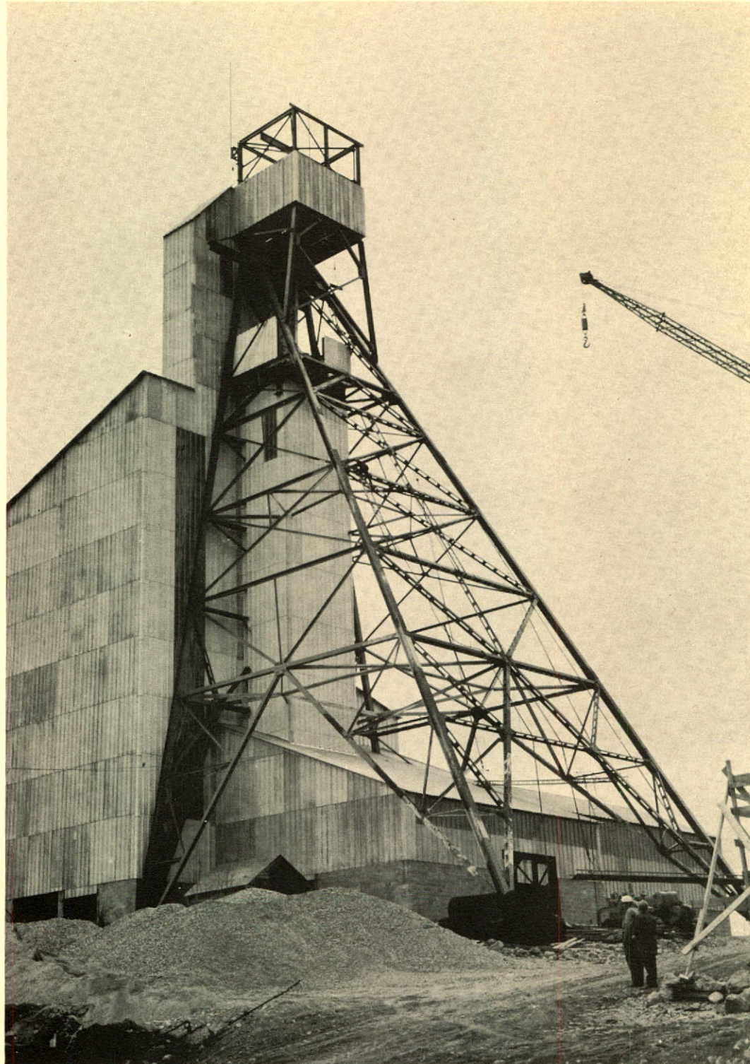
New Quirke headframe under construction preparatory to shaft sinking. This new uranium mine, under development at Elliot Lake, will be phased into production as output at other mines is reduced.
