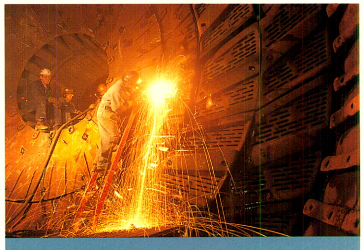
Workers at Highland Valley Copper prepare the interior of the large grinding mill shown on the opposite page.
