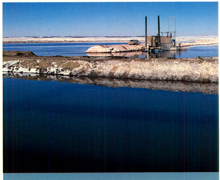
Precipitation ponds under construction at PCA's Saskatoon operations will be used to recover potash extracted by solution mining.
