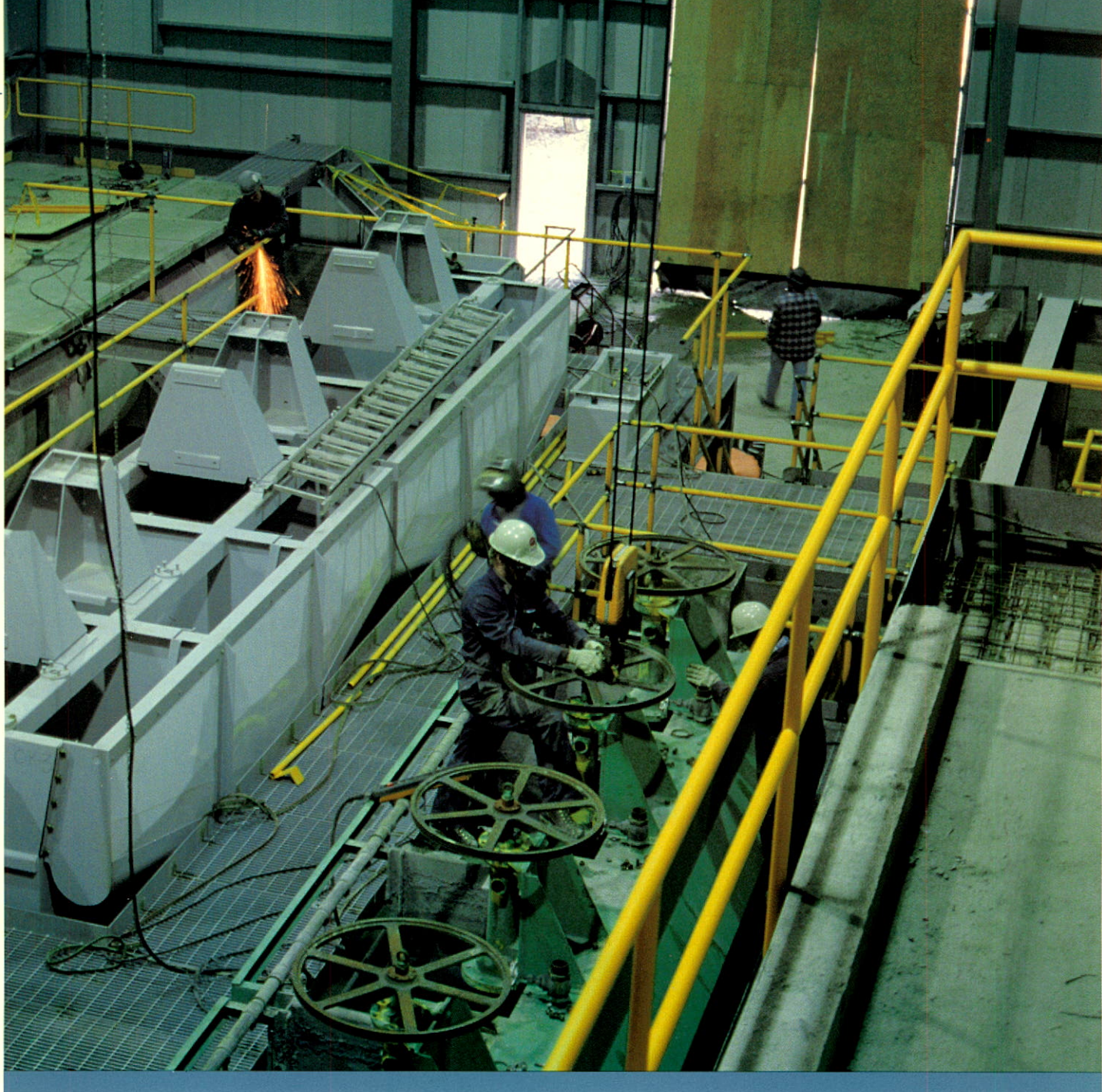
Construction in progress on a new $5.5 million tin flotation circuit at East Kemptville which is expected to significantly improve tin recoveries.
