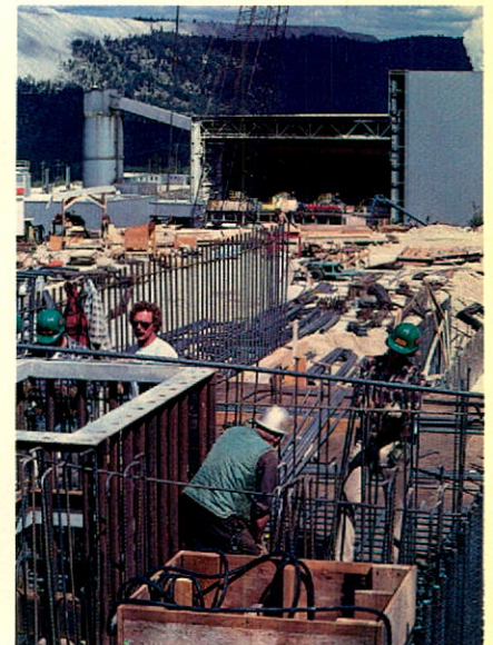
Steel rods and cranes seem to be everywhere as construction proceeds at a fast pace at Lornex.
