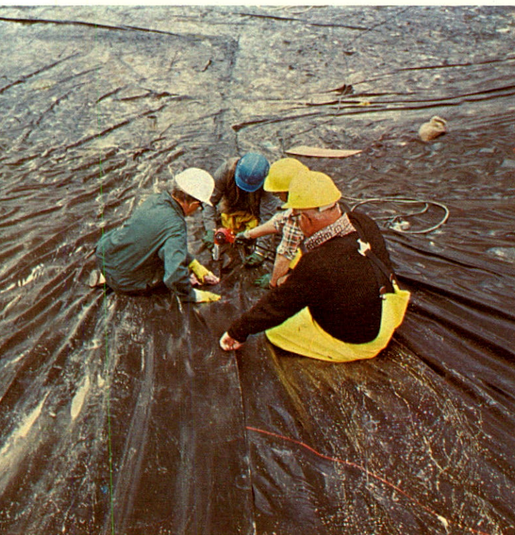
Impermeable vinyl liners are being installed at all Panel mine tailings dams to prevent seepage from containment areas.
