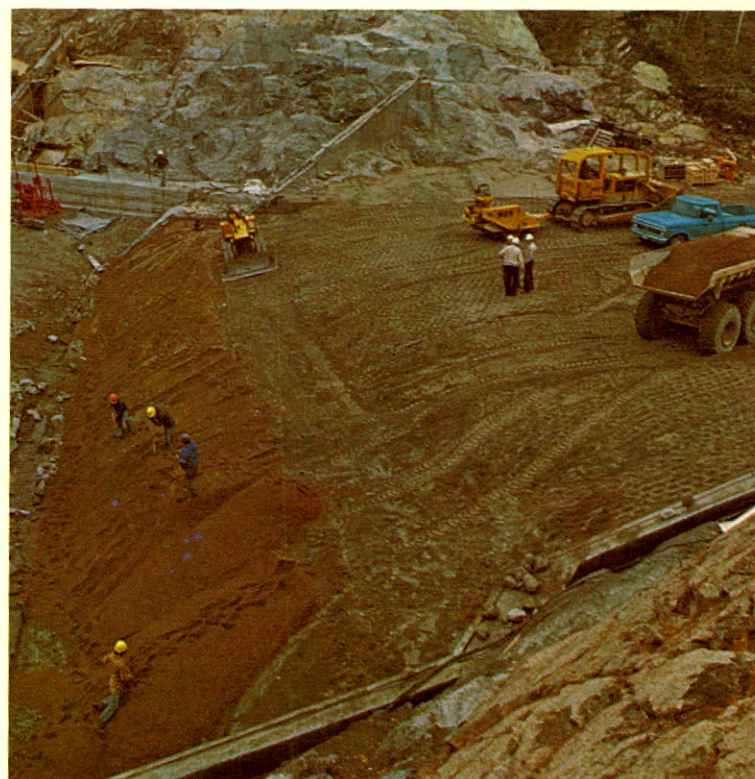
Membranes are seamed (left) and a sand blanket and layer of coarse rock are spread over the liners to prevent them from shifting.
